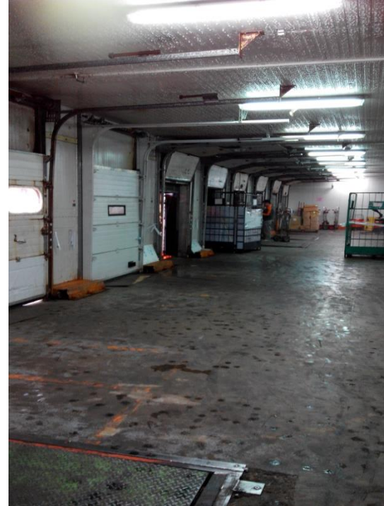
Water stains on floor
