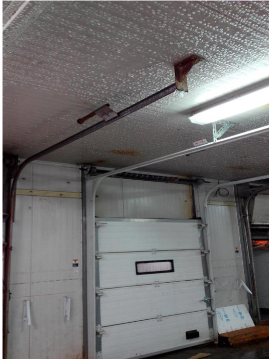
Water drops on ceiling
